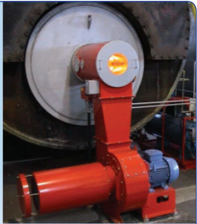
Side : 7.2 ton boiler with Limpsfield burner
