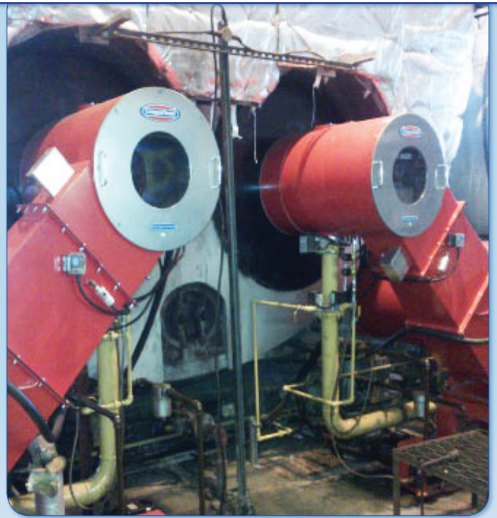
Twin Furnace Boiler
