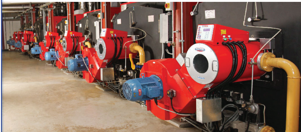
Left: Limpsfield Burners With Integrated Autoflame Combustion Management System
