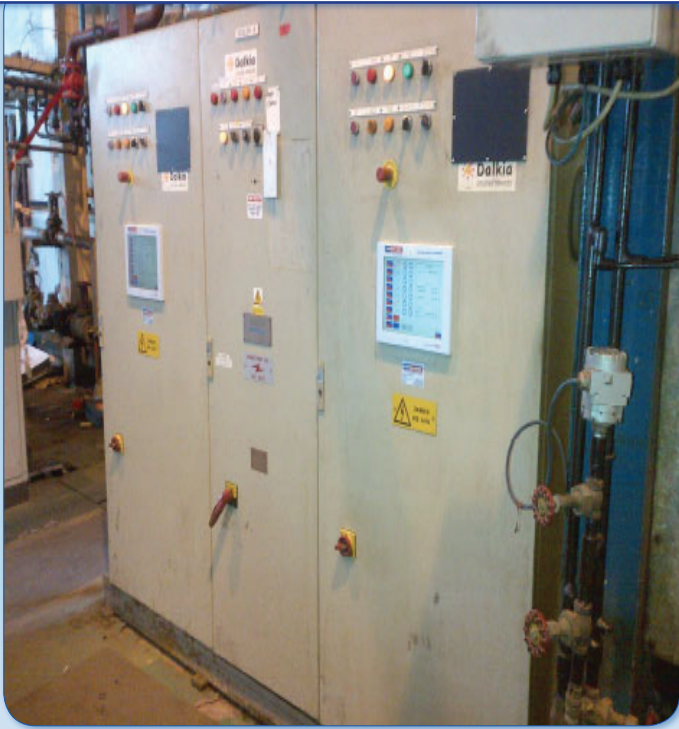
Panel Retrofitted With Mk7 Controllers
